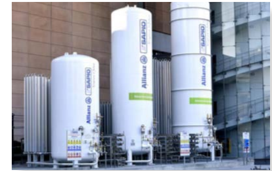
Key learning from the Fiera Milano: plan appropriate fire safety measures when moving, installing and operating (very) large gas and oxygen tanks.
